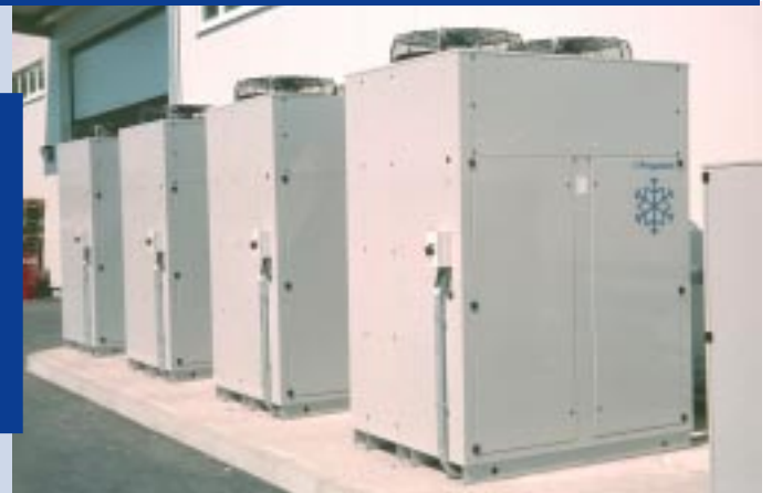
FWC-500 CHILLERS FOR INDUSTRIAL PROCESS COOLING AT MACHINE TOOL SHOP IN EISENACH, GERMANY
