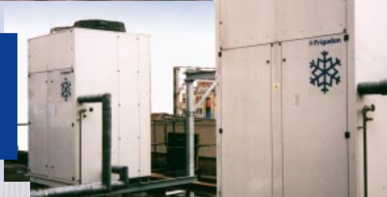
FWC-500-S(3) AIR CONDITIONING CHILLERS INSTALLED AT COOP BANK, LONDON, ENGLAND
