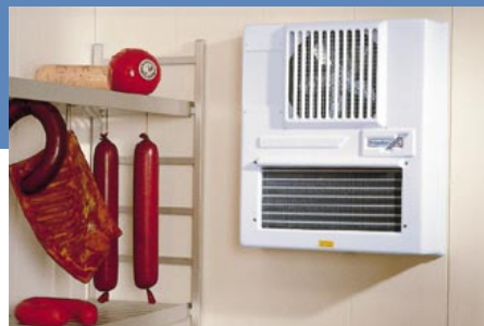
Minicool installed in cold room.
